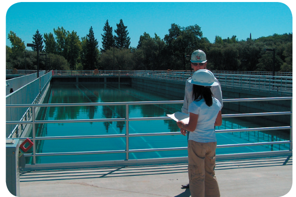
DWR representative Judy Colvin views the City of Roseville's water treatment plant expansion during a recent site visit. City of Roseville Principal Engineer Jim Mulligan provided an overview of the project, one of several that will receive funding under a $25 million Proposition 50 grant for the American River Basin Integrated Regional Water Management Plan.
